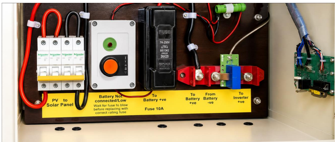
Inside Connection Panel View
